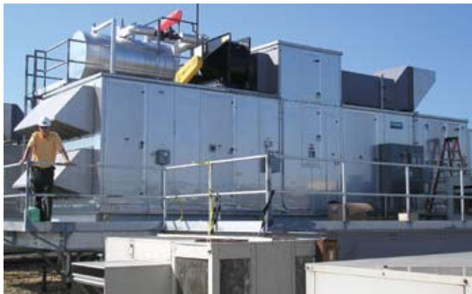
Munters Condensation Control System equipped with PowerPurge™ installed at the Siler City, North Carolina plant.
