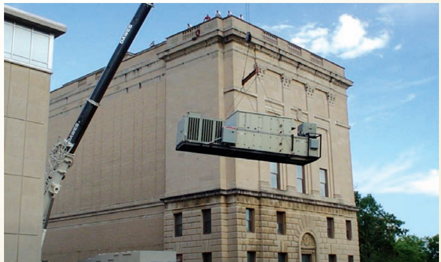
(Above) A crane removes the old dehumidification equipment from the building rooftop. (Top Right) A more efficient and effective Munters humidity control system was installed.
