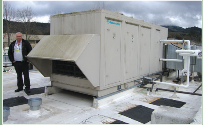
Rooftop units are available in many shapes and sizes, for applications ranging from residential to heavy commercial-industrial. This makeup air unit was placed on top of Sutter Warrack Hospital in Santa Rosa, California.
